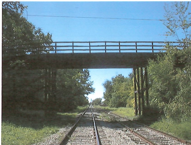
Wood Street Bridge "Major Bridge" Grant to be used for Replacement (City of Shelbyville)
