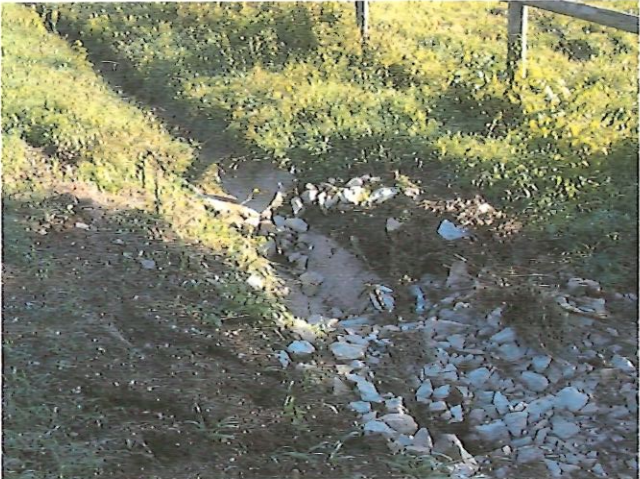
Existing Drainage Gutter Damage
